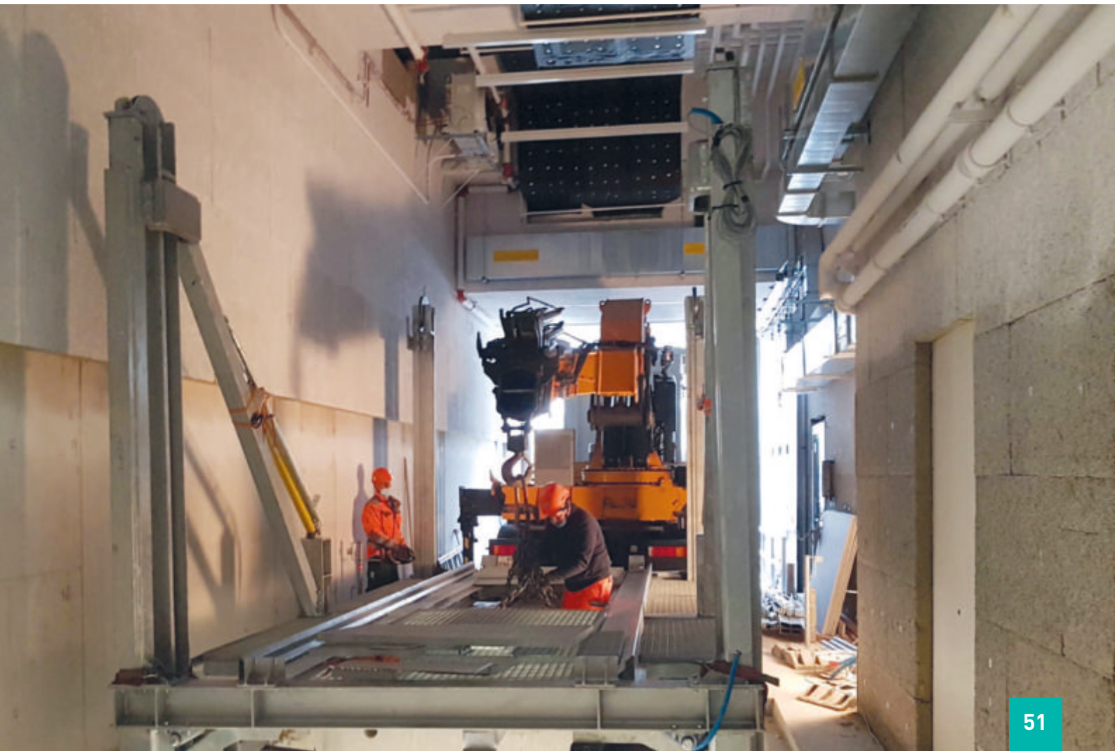
Below: Quadromat lift system installation in the extension complex of a historic building.
