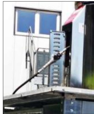
Hydraulic connection to external vehicles
