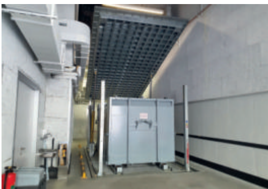
Raised lift for loading the compactor container.
