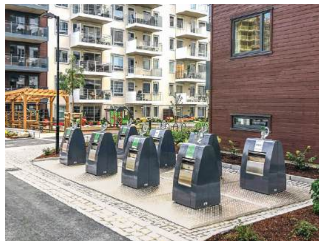
Sub-Vil Lugano with electronic access control and level monitoring.
