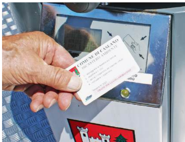
The cover can only be opened via the use of an access card.
